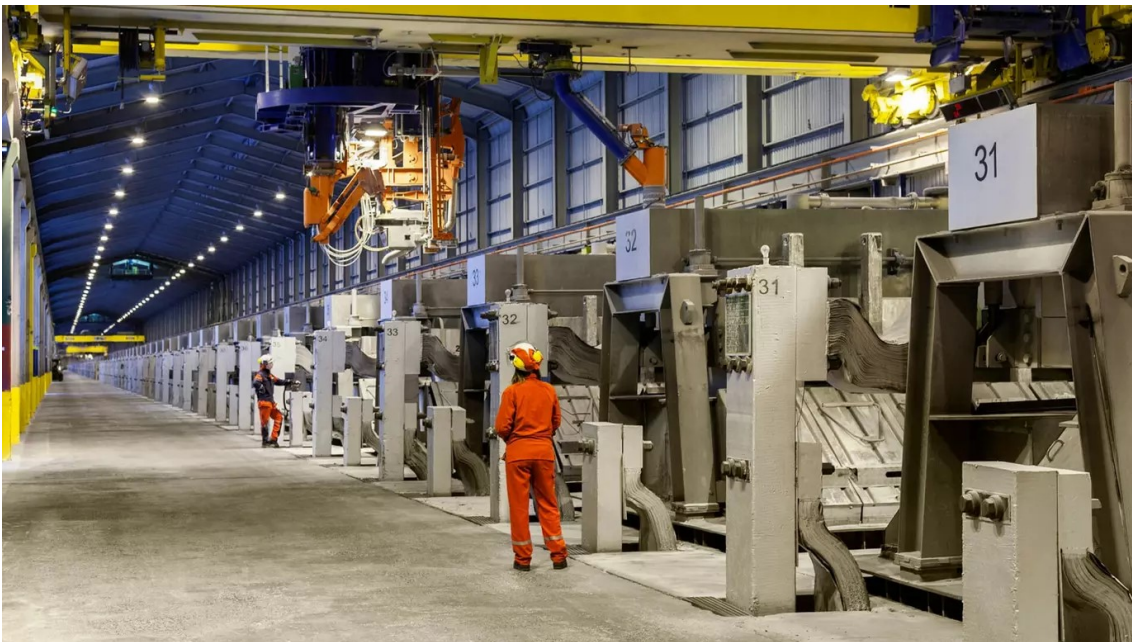
Figure 9. A potroom with VAW's CA 240 cells in Norðurál smelter, Iceland [27].
